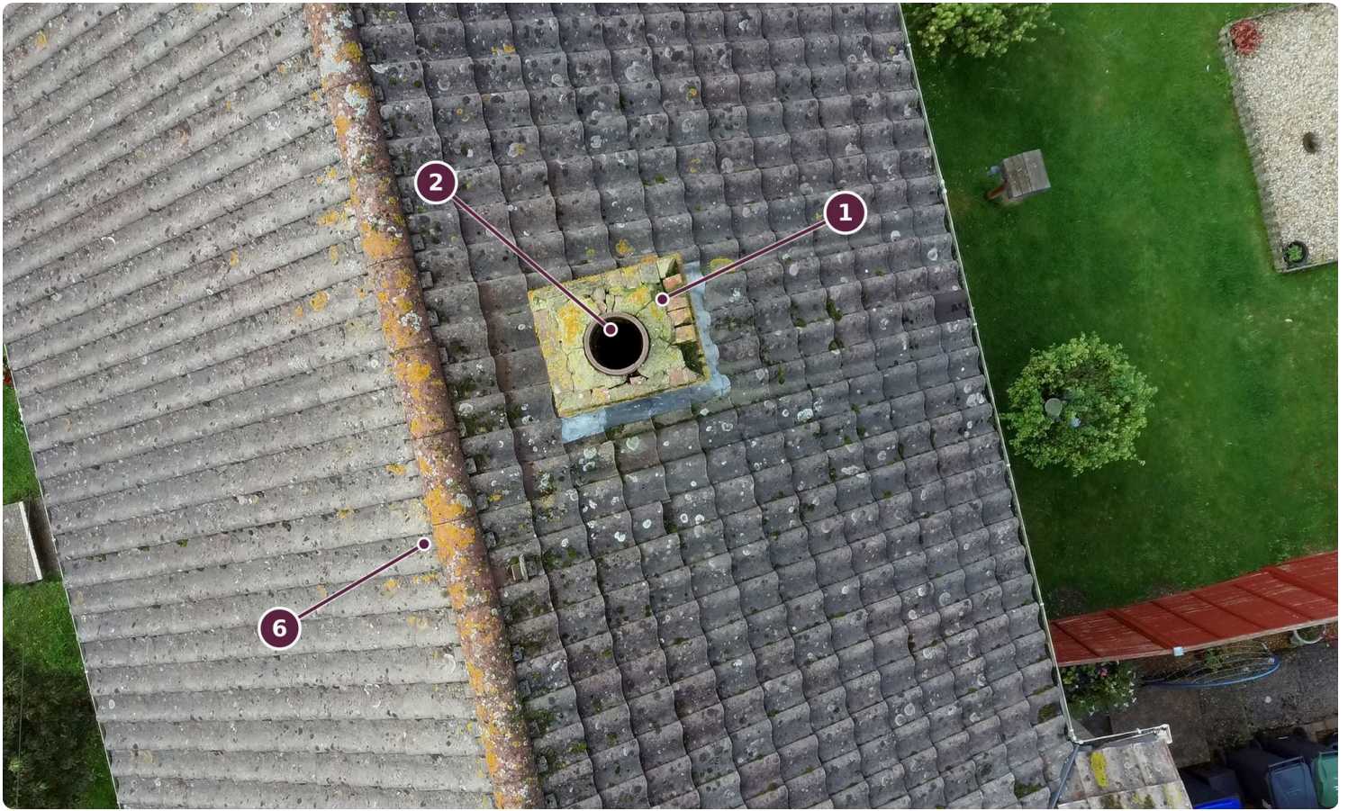
Fig. 1 — directly overhead. The view you cannot get from a ladder. 1 cracked, weathered flaunching around the pot · 2 open pot, no cowl or bird guard · 6 moss and lichen across the tiles and ridge.
