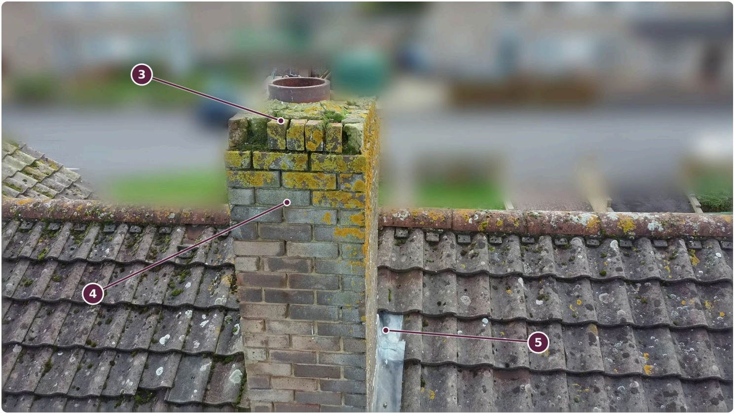
Fig. 2 — at ridge height, front. Close pass on the crown: the displaced coping bricks and moss along the open joints are plainly visible. 3 open joints and vegetation in the top courses · 4 weathered brick faces below the crown · 5 aged but continuous lead flashing at the base.
